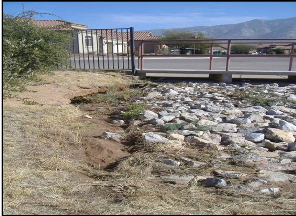
Photo 4.2 Basin Inlet with Inadequate Riprap Placement
