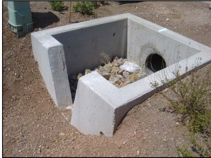
Photo 4.3 Combination Weir Box
